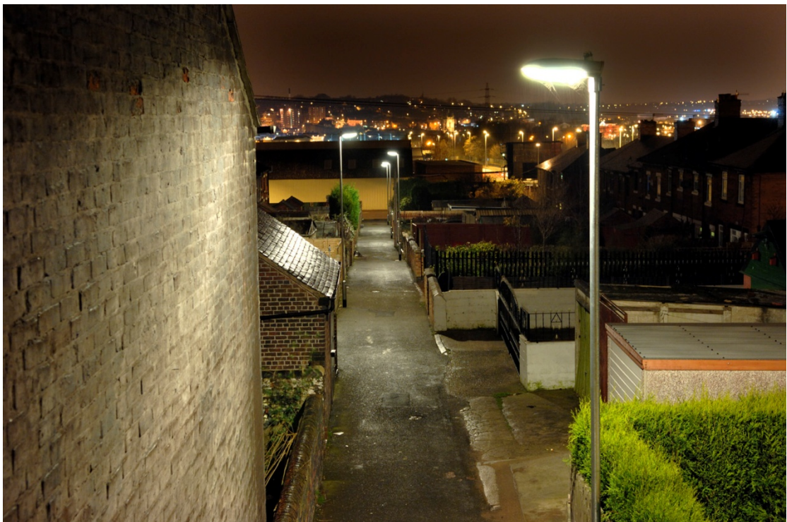
Before and after photos of rear alleyway in Fenton following installation of street lighting. Since the beginning of the PFI programme SSE have lit over 40km of previously unlit back roads.
