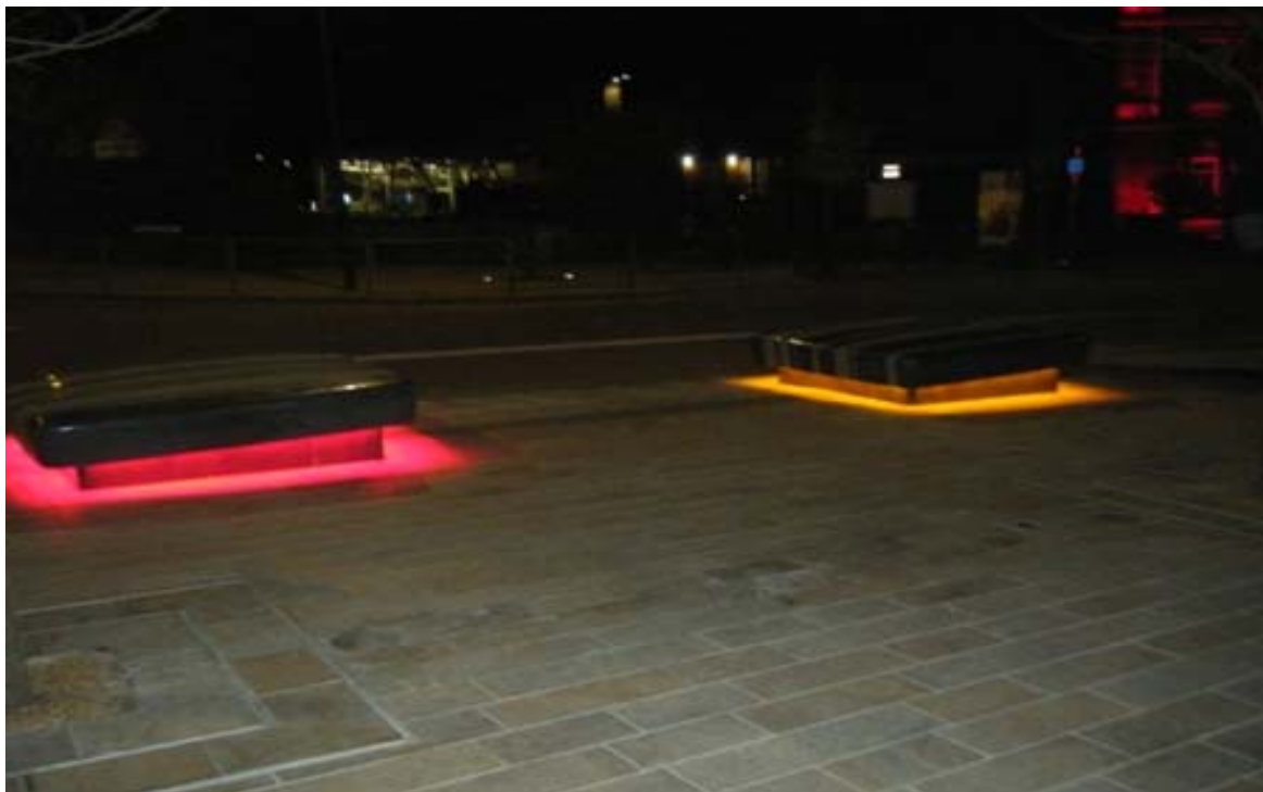
Granite seating bench fitted with LED lighting – installed by SSE.
